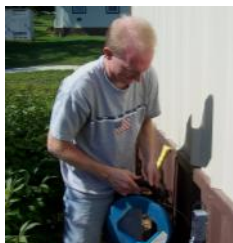
Installing new cables from a classroom building to the new modular building.
